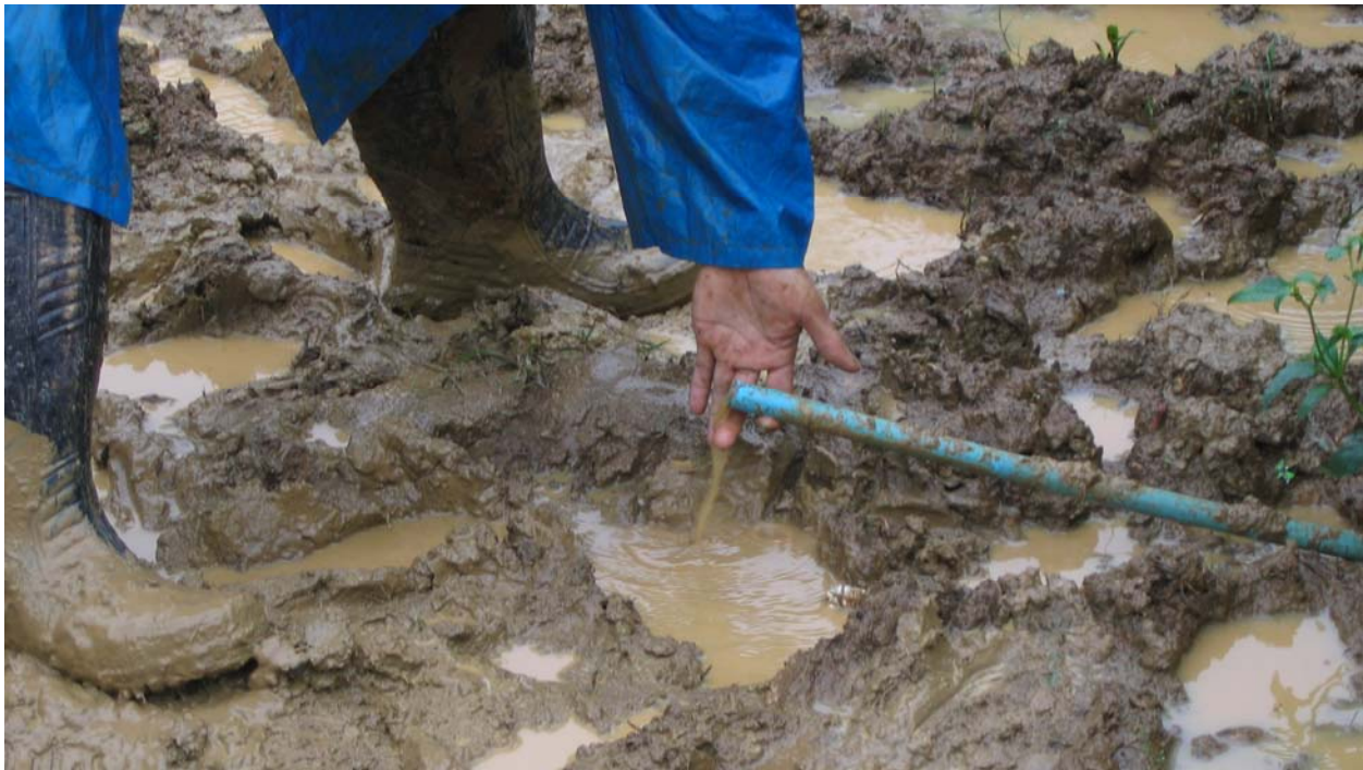
Figure 2: BGET technician Em lifts the broken end of the delivery pipe from the muddy road. Water flows from the break.
