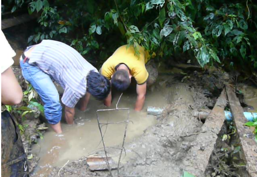
Figure 3: BGET technicians Thai (left) and Sunti (right) stand in the shallow basin and use their hands to remove sediment deposited by run-off from previous rainstorms.
